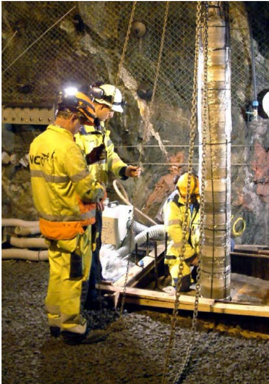
Installation of one of the three packages illustrating the mixing of the different compacted buffer discs.
